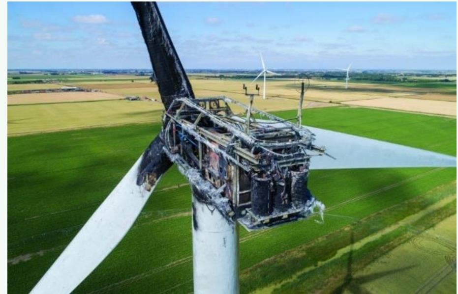
Figure 8- Image of Lightning Damage to a Turbine (Hall, 2021)
